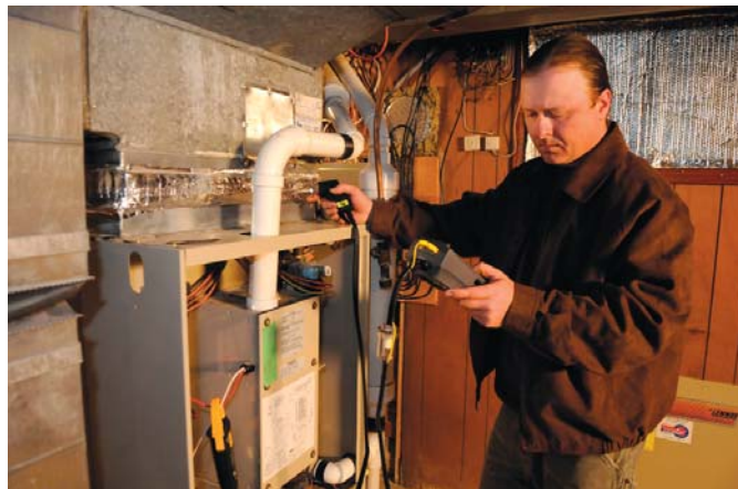
Photo Caption: A CO alarm and an annual heating system inspection is essential to protecting your family from carbon monoxide gas.
